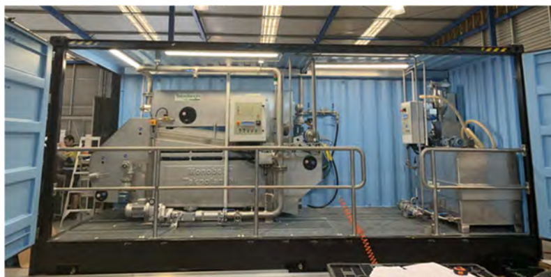
Figure 6 Containerised Monobelt Plant
