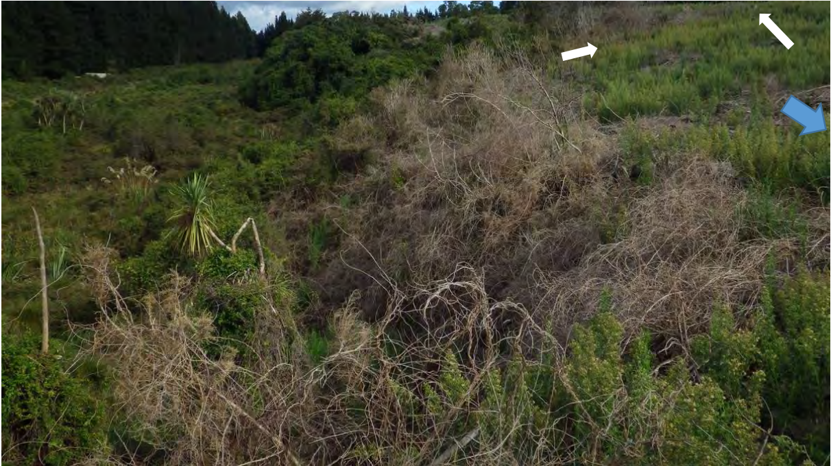
Figure 13 View west from near photopoint 5, showing the extent of the spray damage over the terrace face. Survey pegs are marked with white arrows and the direction to the next survey point with a blue arrow.
