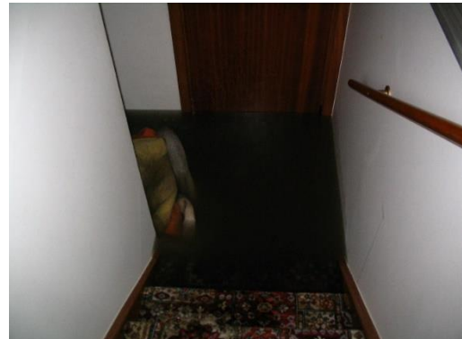
Figure 2: Flooding 01/06/2019 10 School Road Photo 2
