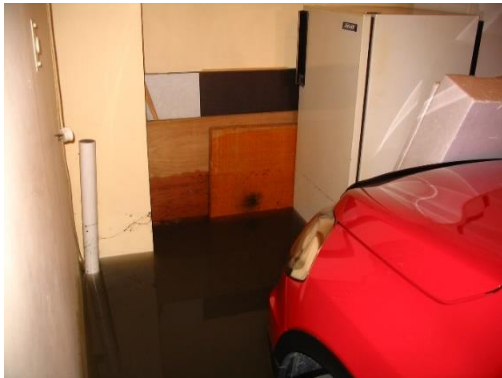
Figure 1: Flooding 01/06/2019 10 School Road Photo 1
