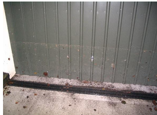
Figure 4: Flooding 01/06/2019 – Water Level 10 School Road Photo 4
