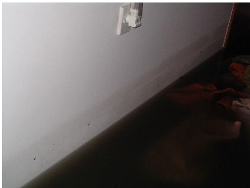
Figure 3: Flooding 01/06/2019 – Water Level 10 School Road Photo 3
