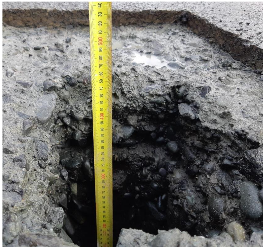
Figure 55: Pothole in Centreline of School Road at Intersection with Gibbs Drive
