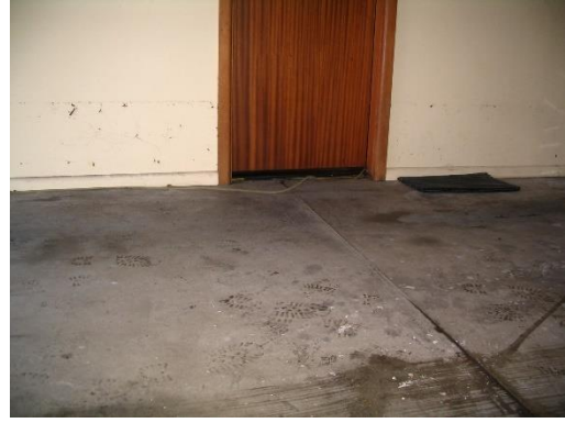
Figure 6: Flooding 01/06/2019 – Water Level 10 School Road Photo 6
