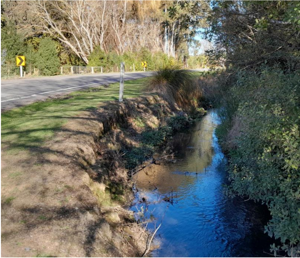
Figure 5: Tuahiwi Stream (Waituere) at Greens Road, showing visible bank erosion, September 2026
