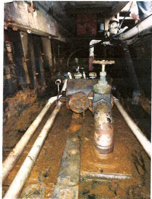
Starboard side old bilge system, some sludge on bottom
