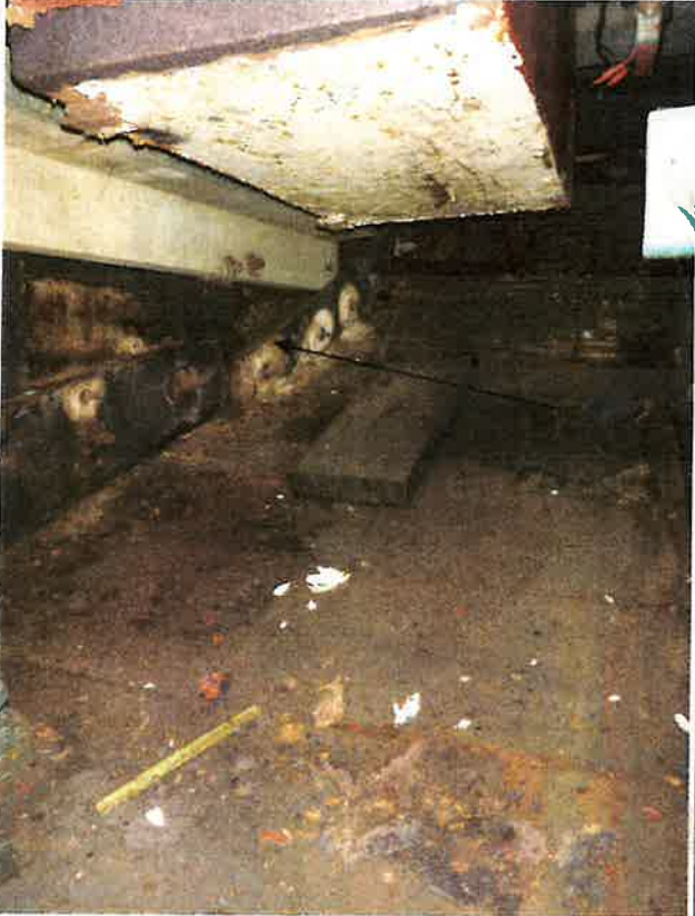
Starboard side aft, soft timber in side of chine.
