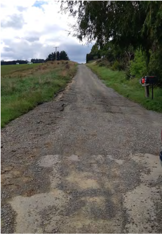
Photo 19 - Doyles Road running course washed off and scour
