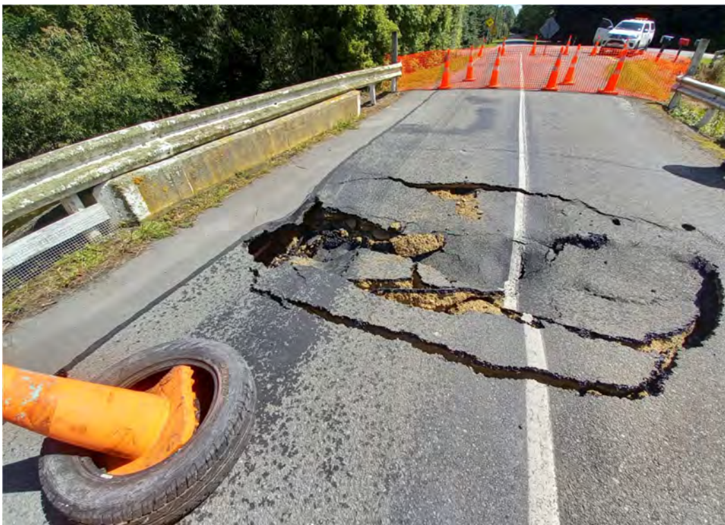
Photo 23 - Butchers Road Bridge Pipe Arch Culvert Collapse
