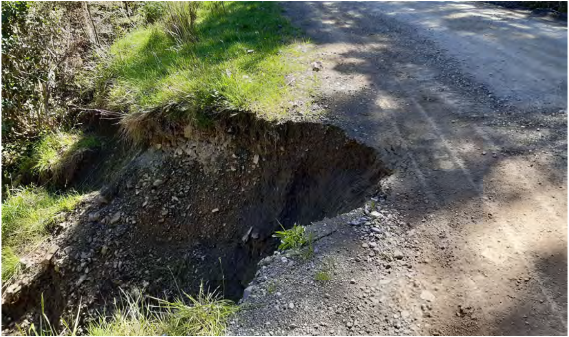
Photo 9 - Lees Valley Rd - Small under-slip (one of four small slips)
