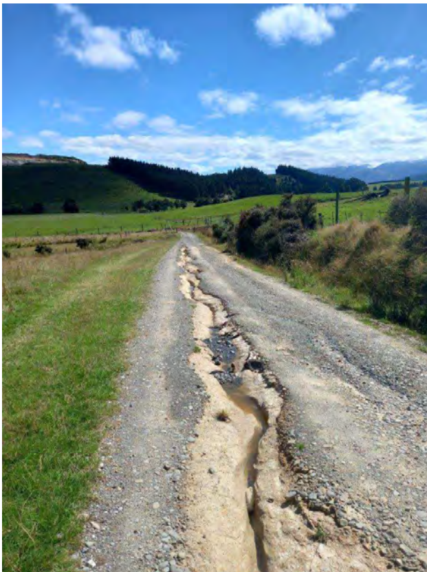
Photo 14 - Wharfedale Track Scour
