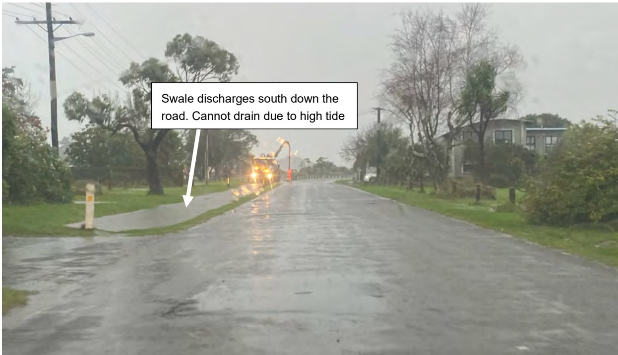
Figure 14: Roadside swales full of water (around 56 Featherstone Ave) (1 May 2025).
