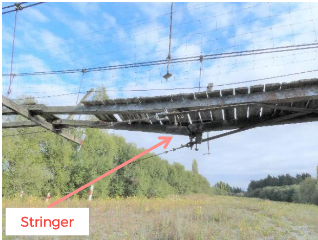
Figure 1.1: Stringer failure near mid-span
