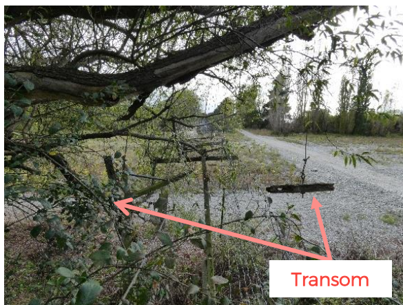
Figure 4.1.5: West abutment transom failure
