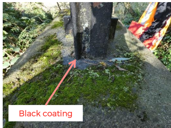
Figure 6.4: Unidentified black coating preventing moss growth on east tower
