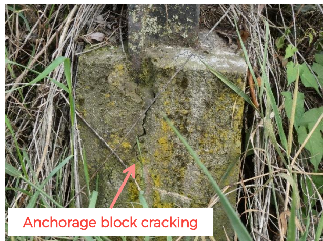
Figure 4.5.4: Cracking in sway cable anchorage block
