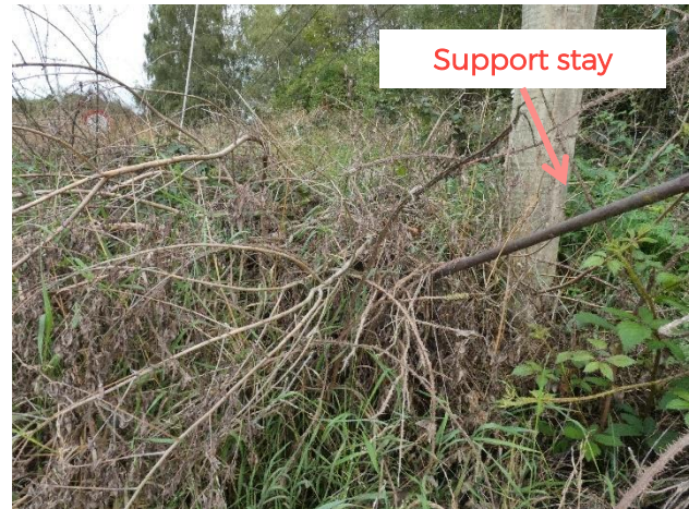
Figure 4.6: Support stay connection obstructed by vegetation
