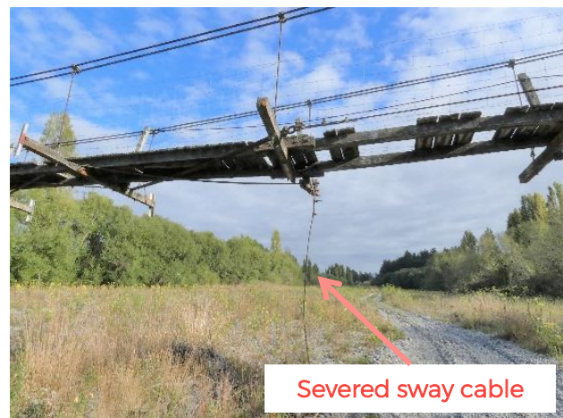
Figure 4.4.2: Severed sway cable – eastern upstream cable
