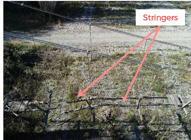
Figure 4.1.4: Stringer failure near east abutment
