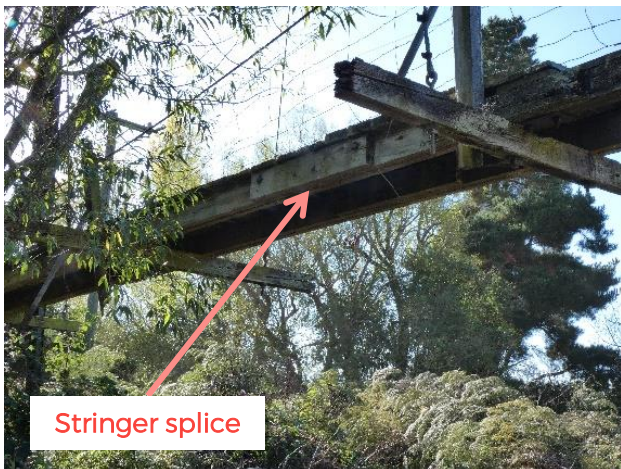
Figure 1.3: Stringer splice condition
