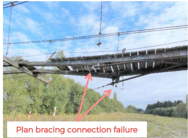
Figure 3.12: Western end of plan bracing - connection failure
