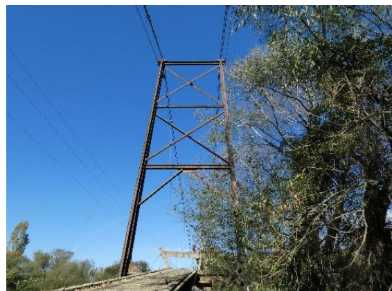
Figure 6.5: Orange colouring to the top of the eastern tower indicates application of unidentified black coating was halted/has worn off the top of the structure
