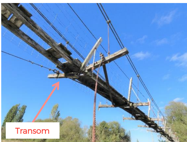
Figure 1.8: Transom failure near sway rope connection
