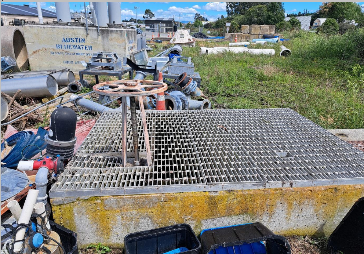
Figure 3: One of the two wet wells involved in the overflow was the eastern wet well shown here. The overflow occurred because one of the two valves in this wet well was closed.
