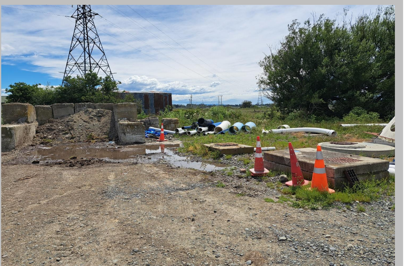
Figure 5: Part of the wastewater overflow from the western wet well was contained by the concrete blocks, while the portion that reached South Brook entered east of the blocks in the pipe-storage area. The liquid visible is screened untreated wastewater.
