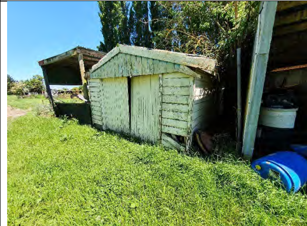
P54: Dilapidated timber garage behind implement shed.
