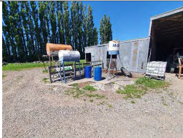
P48: Four petrol and diesel above ground storage tanks (ASTs) located on a concrete pad north of large shed.
