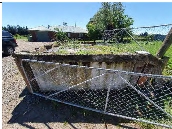
P50: Earthen loading ramp north of ASTs, constructed with soils of unknown origin.
