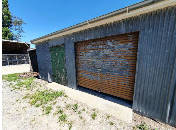
P43: Flaking paint on garage doors.
