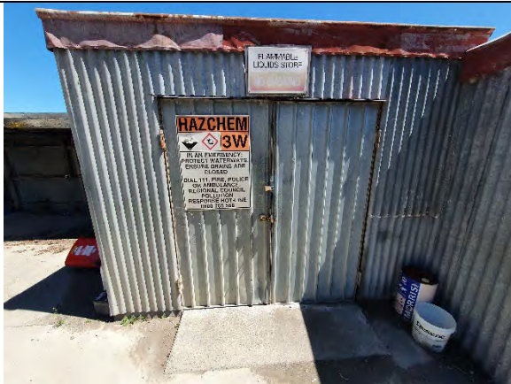
P44: Small chemical storage shed at rear of garage. Could not be accessed at time of site walkover. The paint and oil cans are sitting on a concrete pad.
