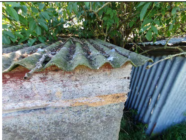
P60: Suspected possible ACM roofing on shed.
