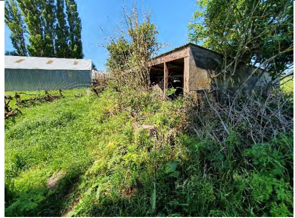
P59: Old shed visible in 1941 aerial. Suspected to have possible ACM roofing.
