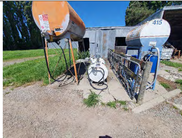
P49: Close up view of ASTs showing some discolouration of ground beneath filling points, indicating minor spillage. Note that concrete show signs of cracking and there are no containment bunds.
