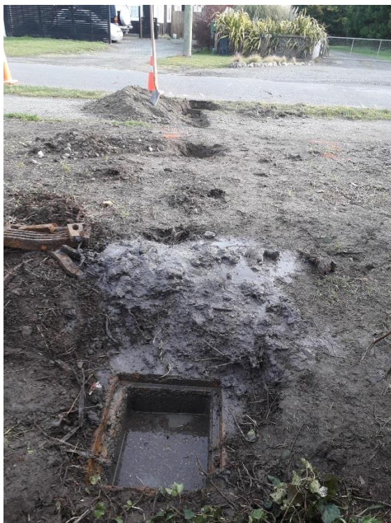
Figure 6. Kings Avenue downstream bubble-up sump opposite 37 / 39 Kings Avenue.
