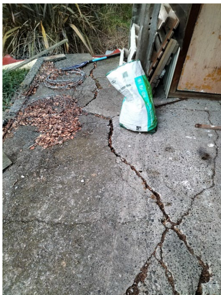
Fig 1.10 a: Cracked Slab on 290 Bradleys Road
