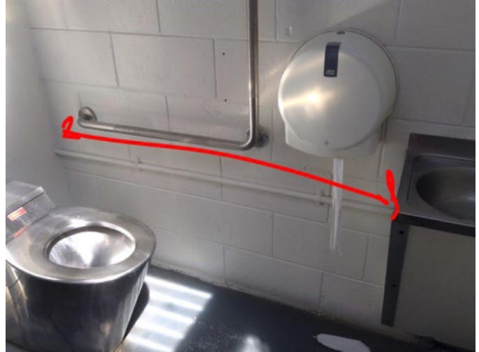
Toilet roll holder too far from toilet – Woodend town centre
