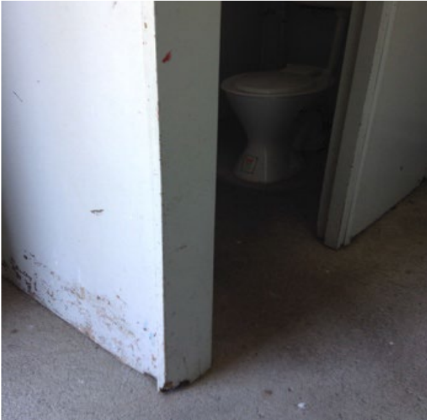
Poor condition of toilet interior walls at Warren Community Reserve
