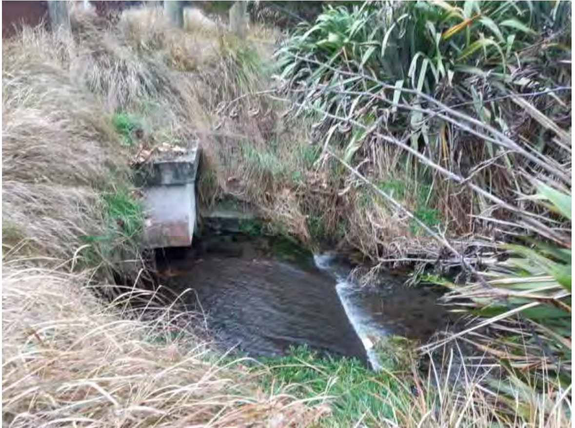
Figure 1: Likely partial fish passage barrier on a North Brook tributary – Corner of Cotter Lane and Northbrook Road
