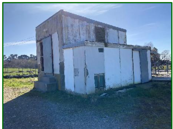
Photo 13 – Dairy with broken cement board cladding
