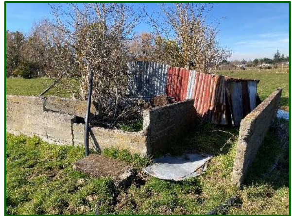
Photo 21 – Derelict animal shelter/shed
