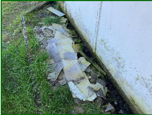
Photo 14 – Pieces of broken cement board on ground
