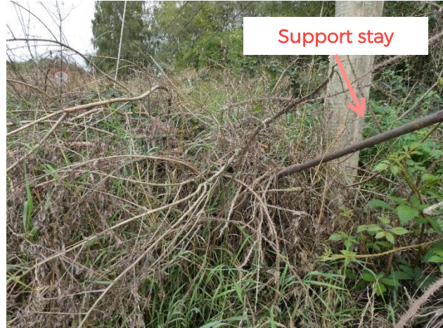
Figure 4.6: Support stay connection obstructed by vegetation
