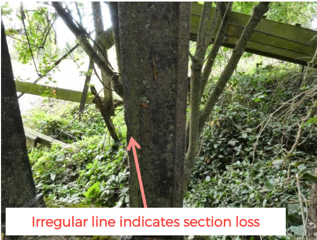
Figure 5.3: Tower steel member - indication of minimal section loss - western tower
