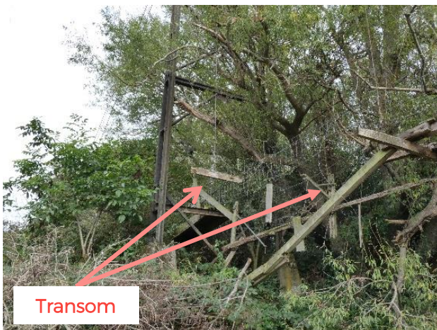
Figure 1.6: West abutment transom failure
