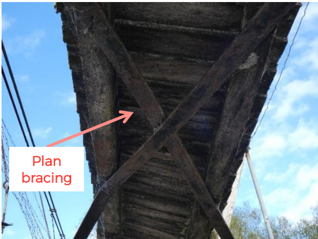
Figure 3.11: Surface corrosion on steel plan bracing flat plate
