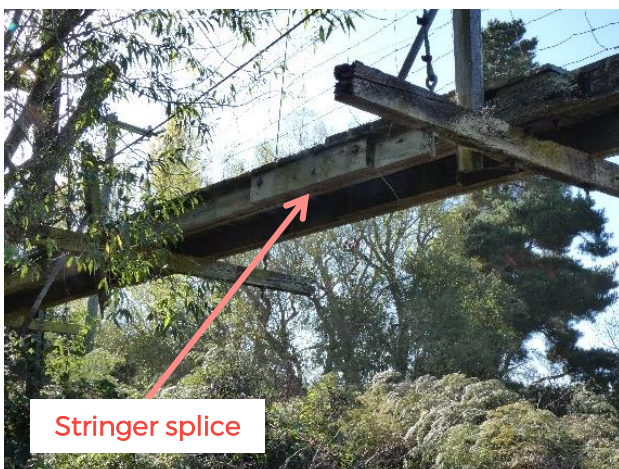
Figure 1.3: Stringer splice condition
