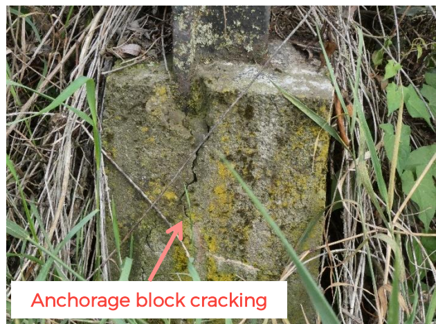
Figure 4.5.4: Cracking in sway cable anchorage block
