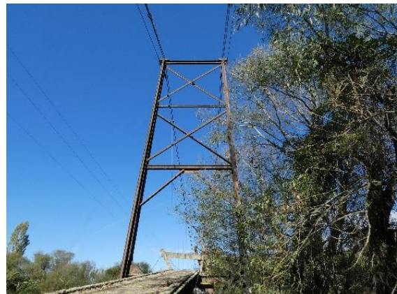
Figure 6.5: Orange colouring to the top of the eastern tower indicates application of unidentified black coating was halted/has worn off the top of the structure
