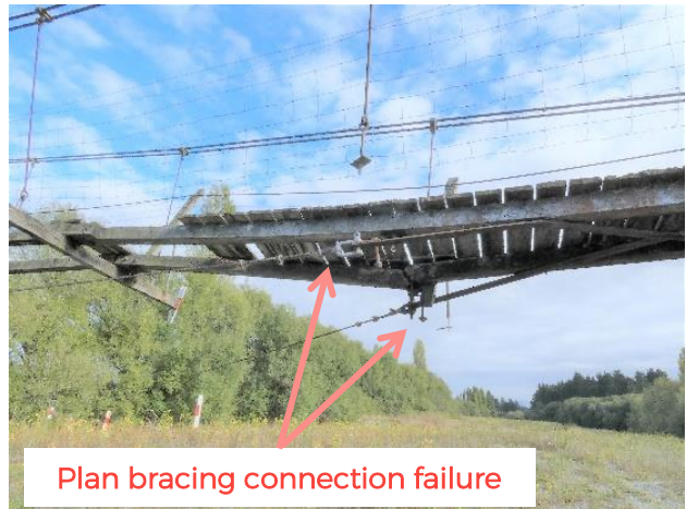
Figure 3.12: Western end of plan bracing - connection failure
