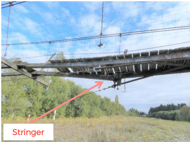
Figure 1.1: Stringer failure near mid-span
