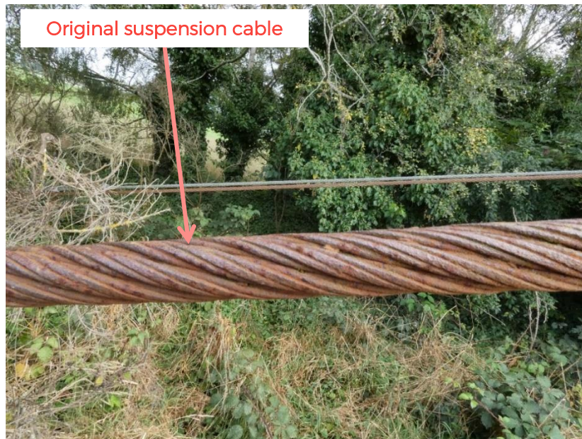
Figure 4.3.3: Surface and pitting corrosion on west abutment downstream original cable
