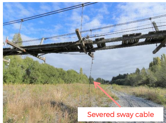
Figure 4.4.2: Severed sway cable – eastern upstream cable
