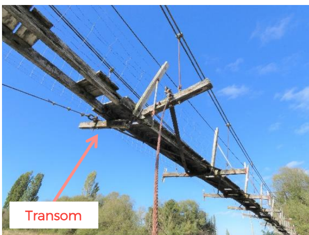
Figure 1.8: Transom failure near sway rope connection
