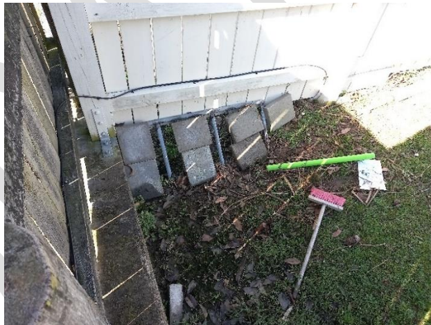
Figure 8: Concrete Blocks Blocking Swale Outlet
