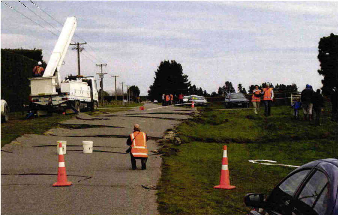
Figure 3 A strike-slip fault offset produced by the Greendale Fault rupture (Selwyn District) during the Darfield Earthquake, 4 th September 2010. This scene was photographed on 5 th September looking south-southwest along Highfield Road, about 8 km west-northwest of Burnham and 0.5 km north of the Highfield Road/Grange Road intersection. The fault rupture here comprised a ~40 m wide zone of fractures, across which the ground was shifted to the right (right-laterally) about 4.5 m, more than half the width of the tarseal, and the far side was bulged up by about 1 m. Prior to the fault rupture, the road was straight and the ground was flat. Photo: D.J.A. Barrell, GNS Science.
