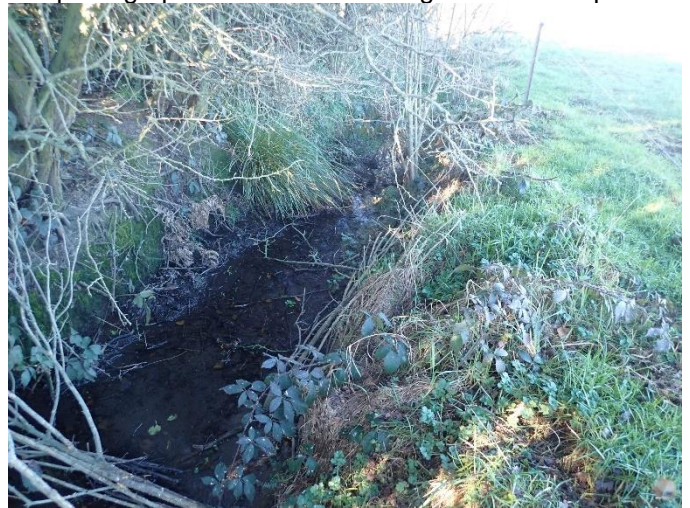
Figure j. Ponded drain, downstream of the GM set. Note the absence of aquatic flora.
