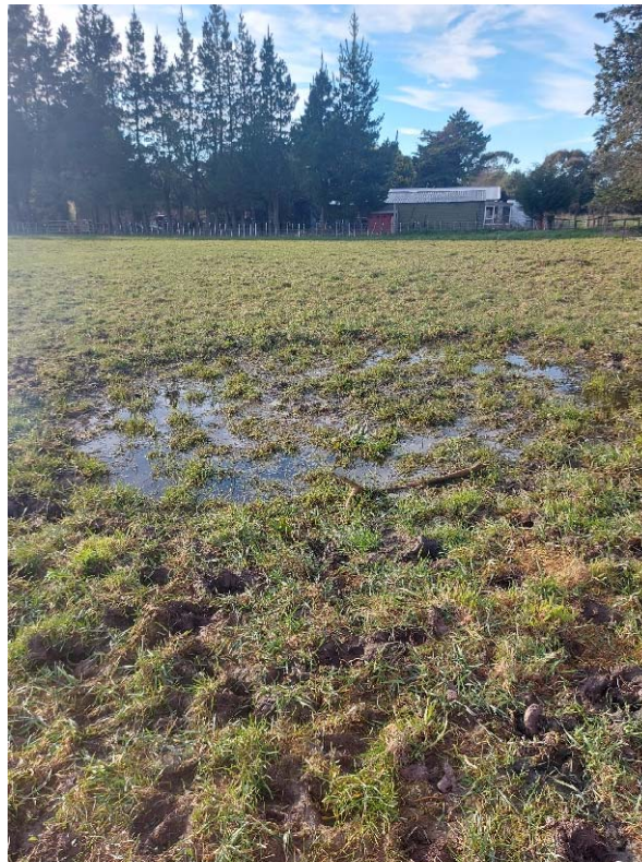
Figure 2: Surface water ponding in a depression area.
