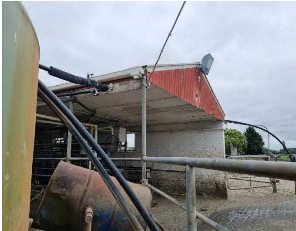
Photo 11: Asbestos in a degraded condition was observed on a milking shed along the eastern boundary of the site.
