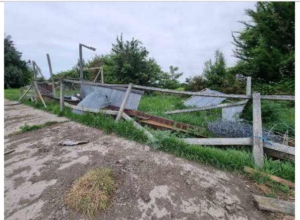
Photo 14: Remnants of an old barn / structure along the north-western side of the site.
