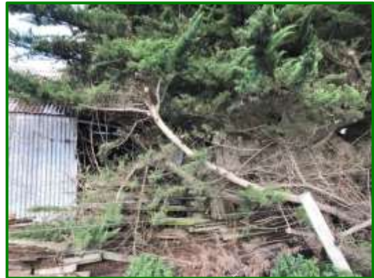
Photo 14 – Derelict timber and iron woolshed
