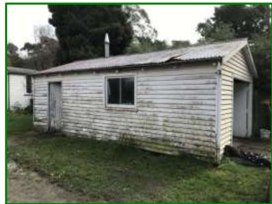
Photo 2 – Poor condition paint on garage
