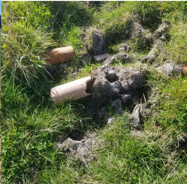
Image 4B Clay tiles damage at south end of site.
