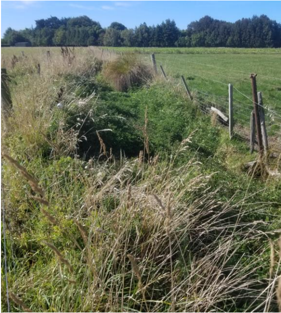
Image 4A Open drain looking NNE
