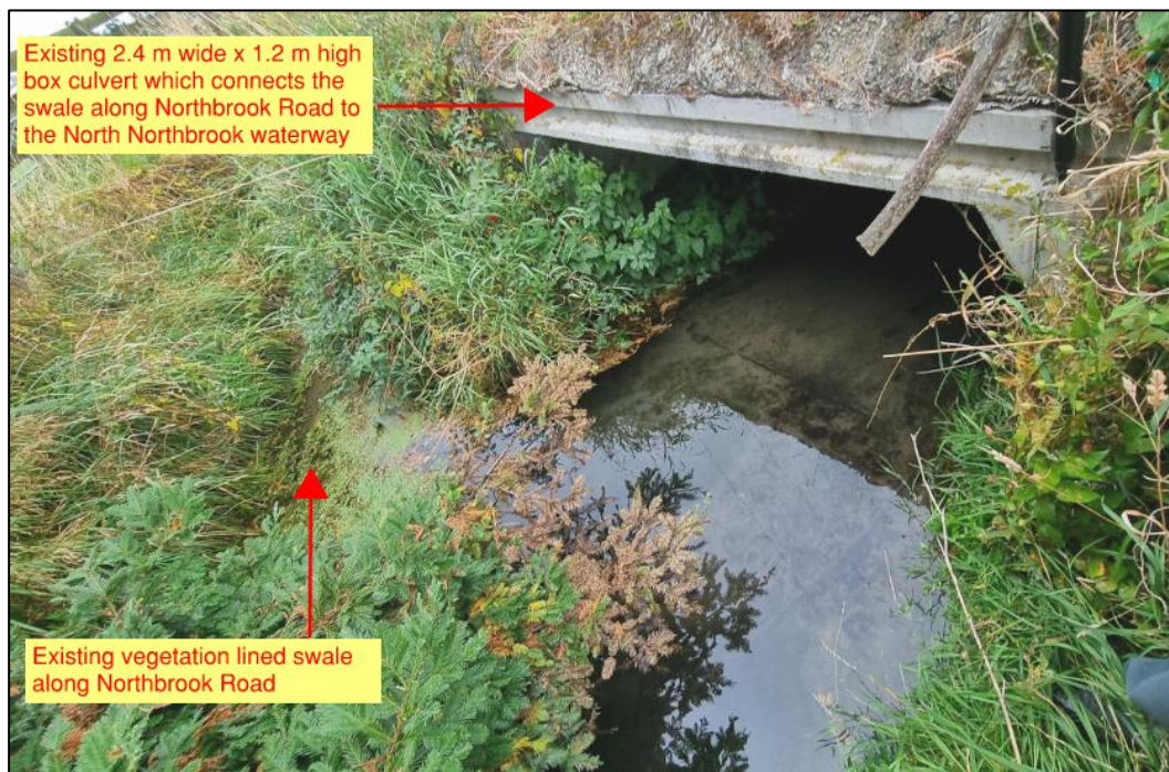
Figure 11 Existing vegetation lined swale and 2.4 m x 1.2 m box culvert along Northbrook Road which connects the swale to the downstream North Northbrook waterway (image taken from onsite investigation)
