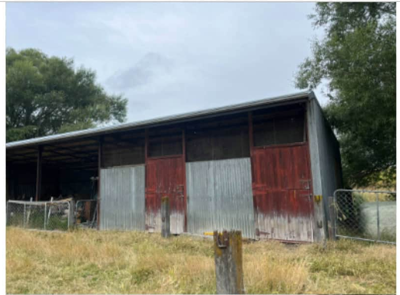
16. Barn in paddock at 144 Main North Road
