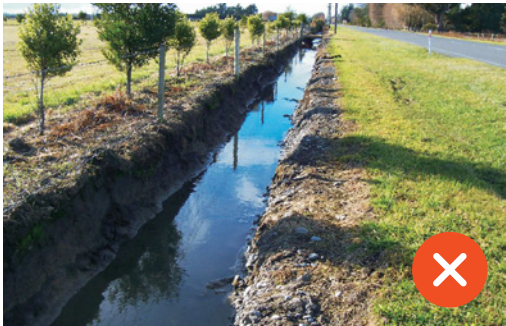
Herbicide spray causing unstable banks
