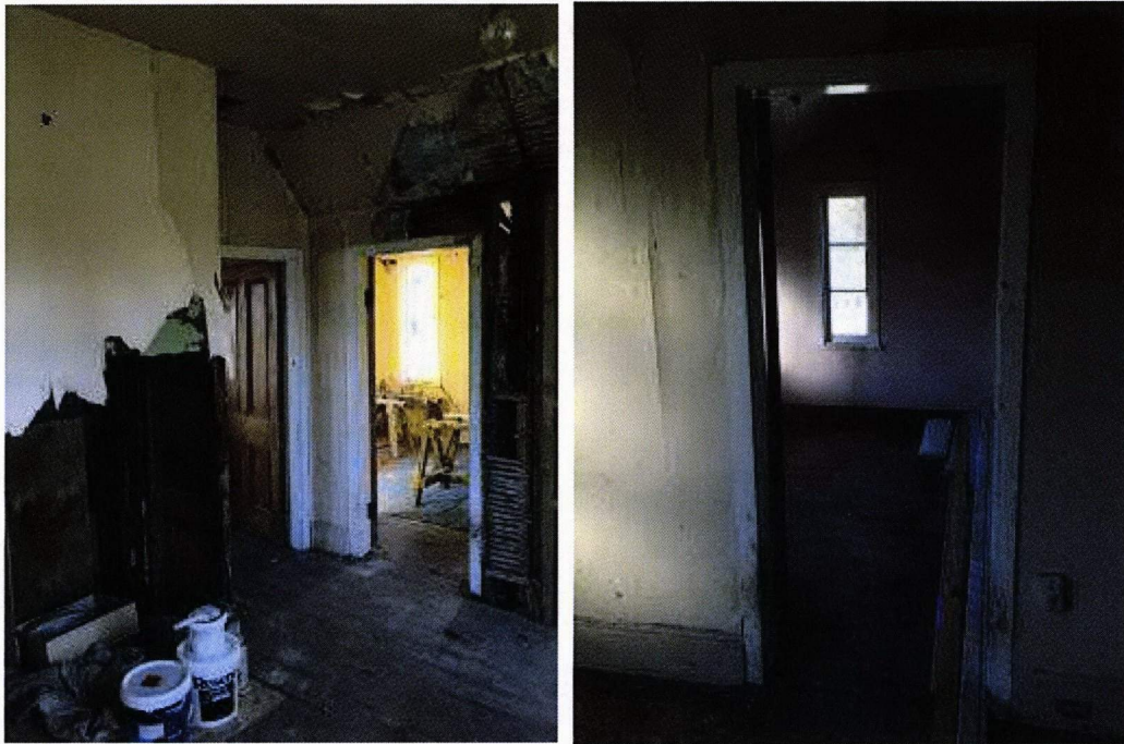
Photos showing the interior awaiting repair (R. Burgess, 9 July 2019, Heritage New Zealand)
