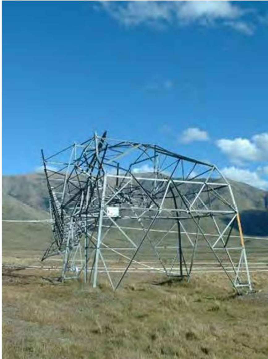
Figure 25: Failed tower on the Benmore-Haywards A line
