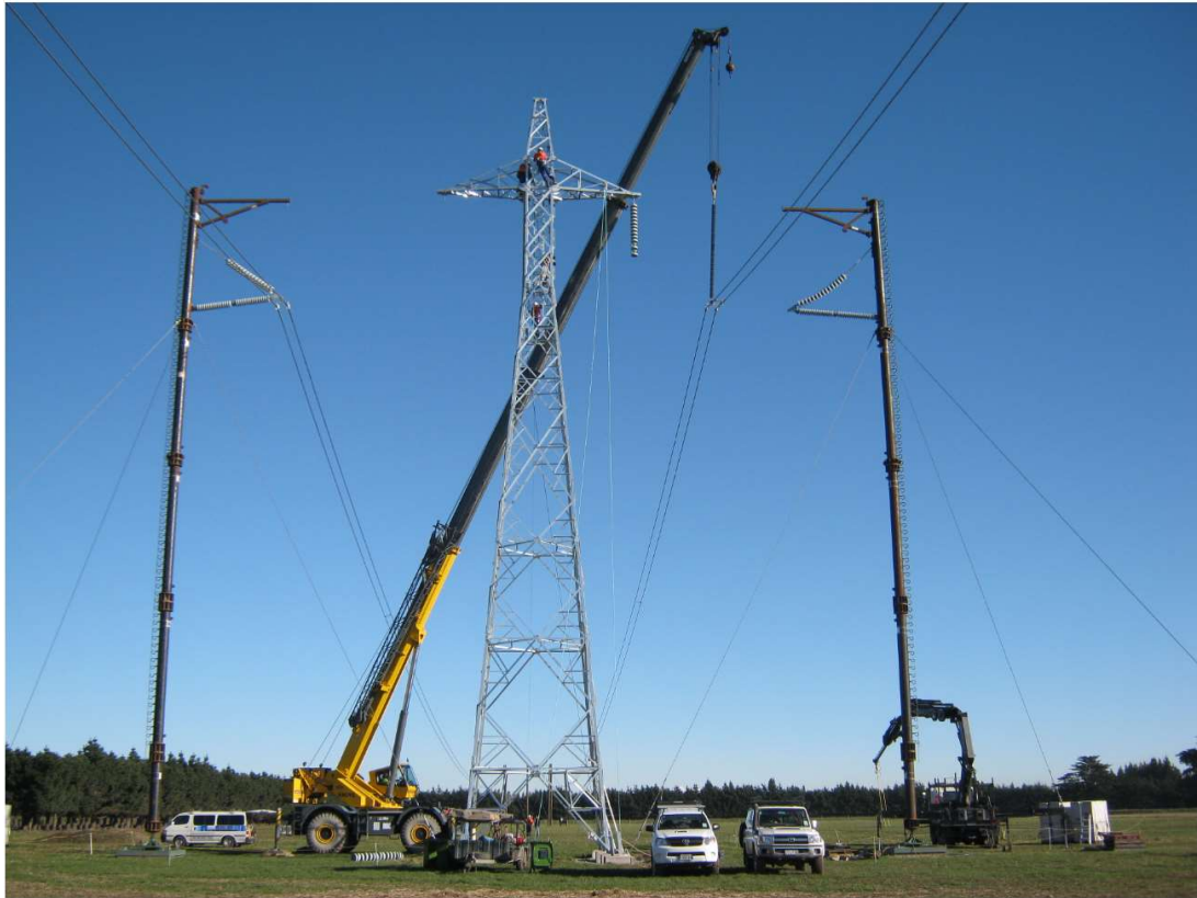
Figure 19: Example of access and construction space required on the HVDC line. Installing more structures on the line.
