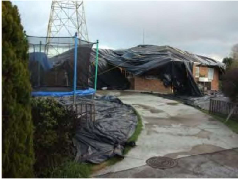
Figure 4: Tower painting in an urban setting, note the extensive polythene sheet protection
