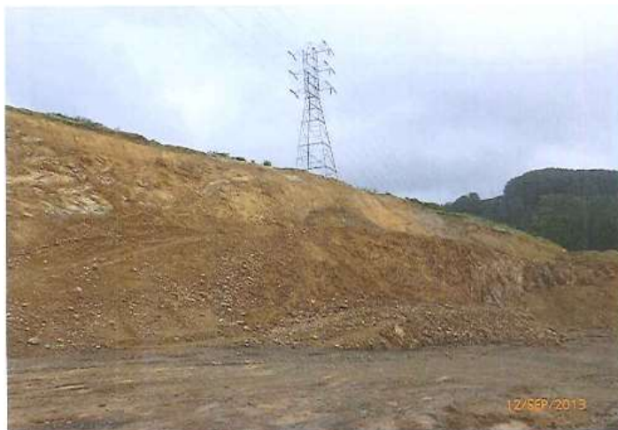
Figure 27: Earthworks in Porirua compromising the foundations of the tower
