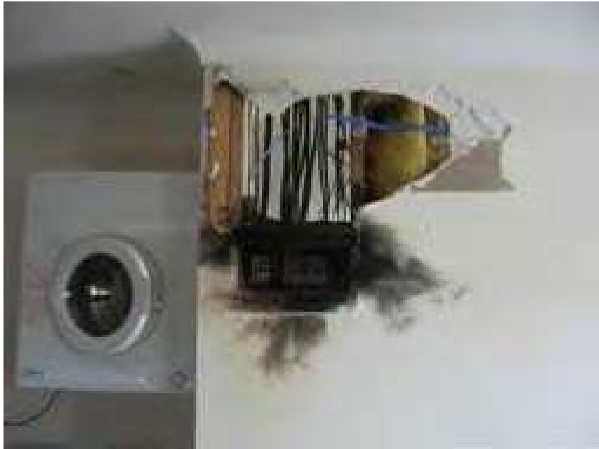
Figure 22: Electrical damage following a conductor drop
