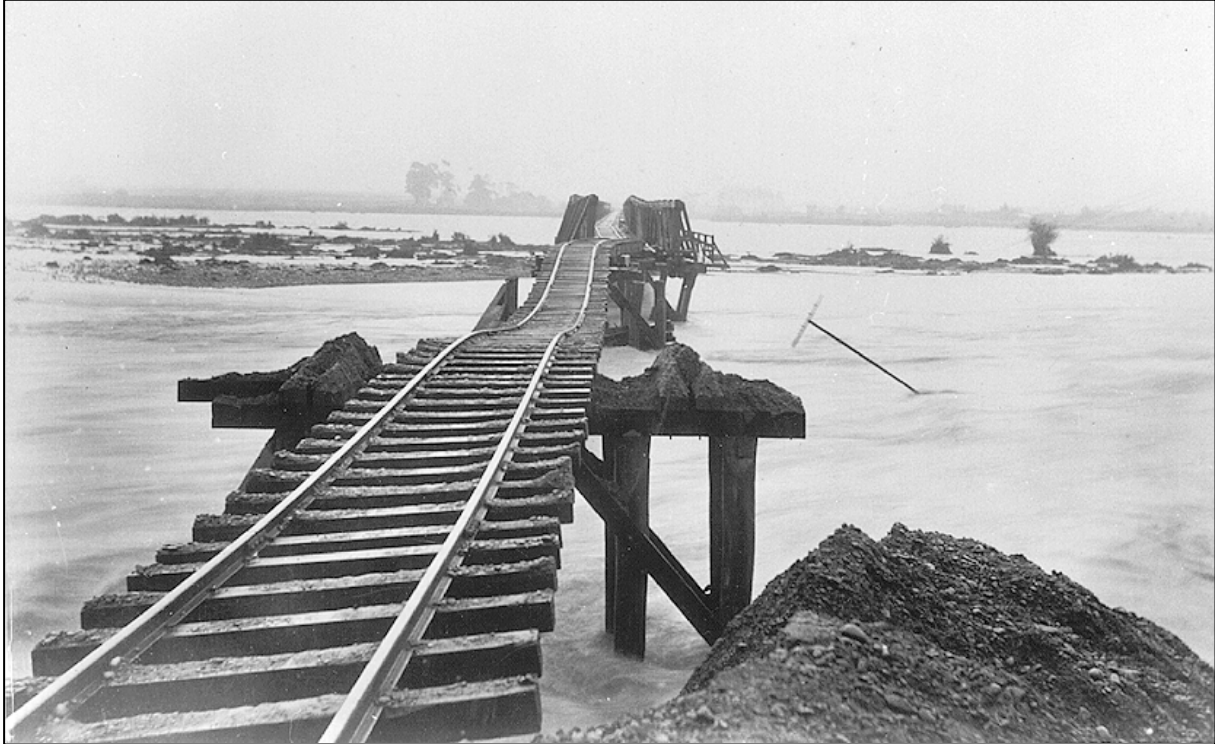
Figure 2-1: Damage to the Ashley River railway bridge in the March 1902 flood
