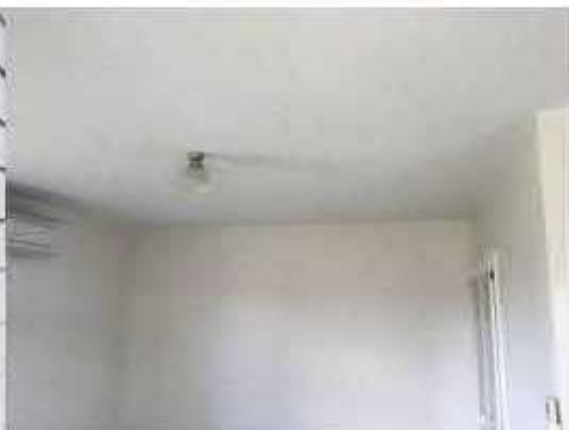
Figure 10: Stippled ceiling plaster in the more recent residential dwelling (possibly containing asbestos).
